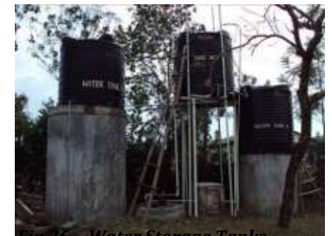
Fig 26 - Water Storage Tanks
